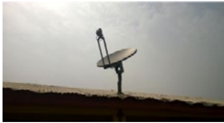
Satellite dish installed on a remote school roof
