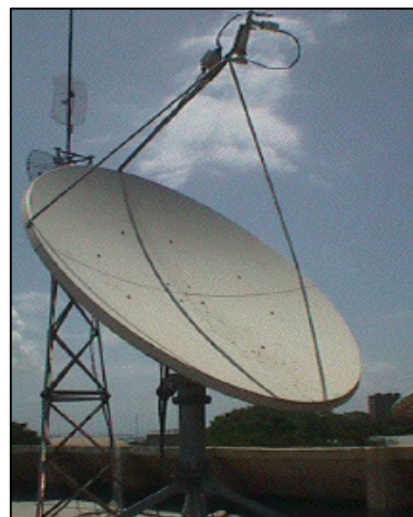
VSAT installation, University of Dar es Salaam
